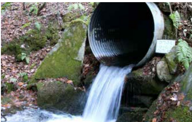
Figura C8. 6. Alcantarilla perchada o elevada. Fuente: Massachusetts Stream Crossing Handbook (Division of Ecological Restoration, 2012) .
